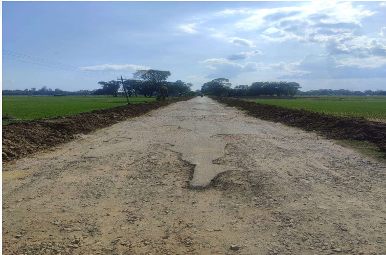
Highly Distressed/Base or Subbase Failure
