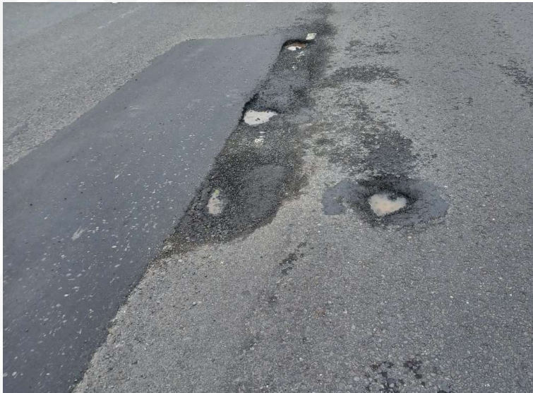
Series of Potholes
