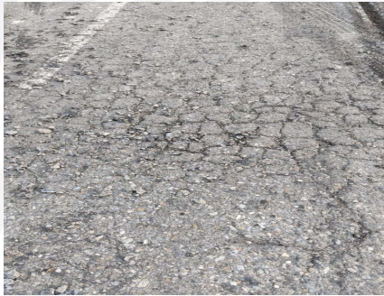
Distressed Existing Surface
